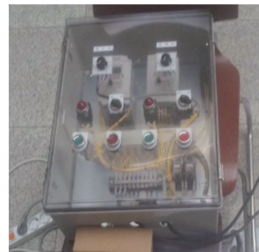
(b) Control box
